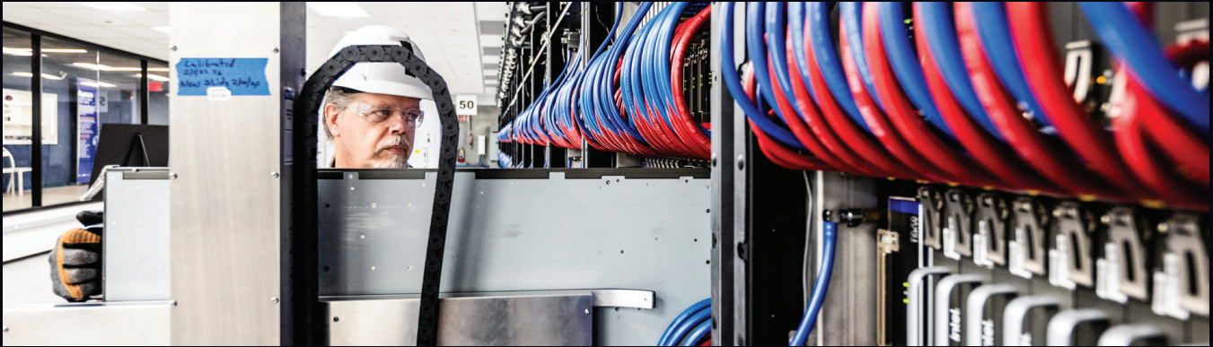
A technician uses a specialized machine to install compute blades into the Aurora system.
